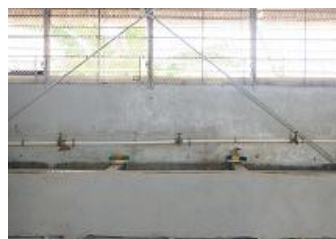
Concrete Wash Tank
