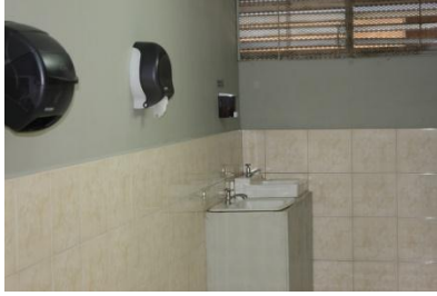
Figure 13 Typical Hand Wash Facility
