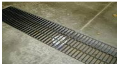
Figure 7 Open Drain Having Suitable cover to Prevent Entry of Rodent
